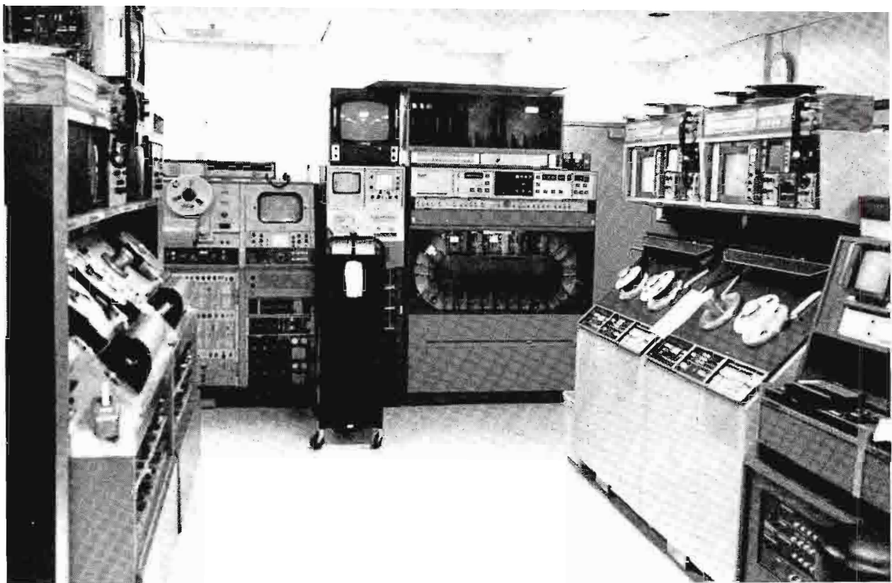
Video Tape area adjoins Master Control. MC operator also loads "cart" machine.
