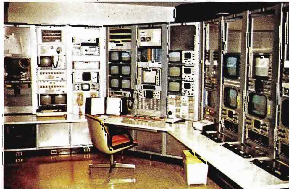
Customized Master Control grouping, with transmitter/STL monitoring facilities on left; switching and machine controls in center, and camera CCU's at right.
